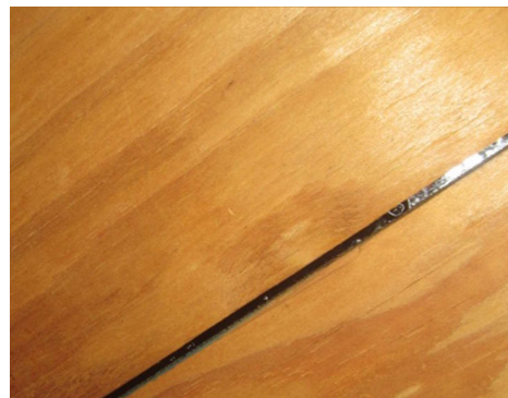
SWR installed under covering
