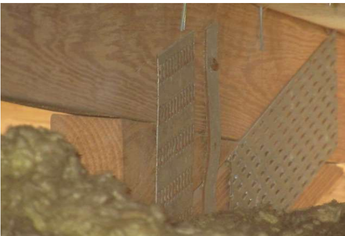
Single strap with 1 nail into the truss
