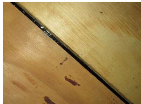
SWR installed under covering
