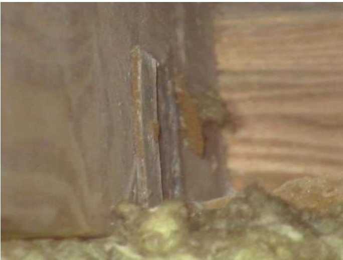
Single strap with 1 nail into the truss
