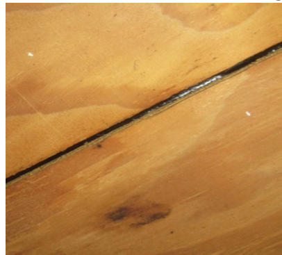
SWR installed under covering
