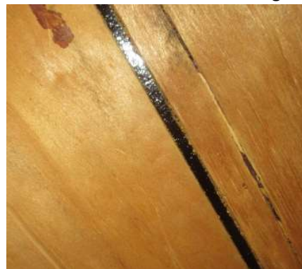
SWR installed under covering
