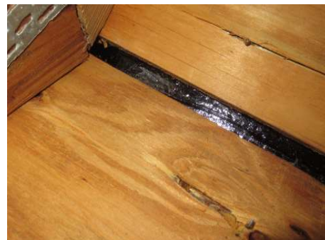
SWR installed under covering
